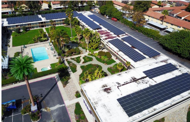
Ramada Silicon Valley recently installed a 269 kW photovoltaic system with 996 Mitsubishi Electric Diamond Premium modules.
