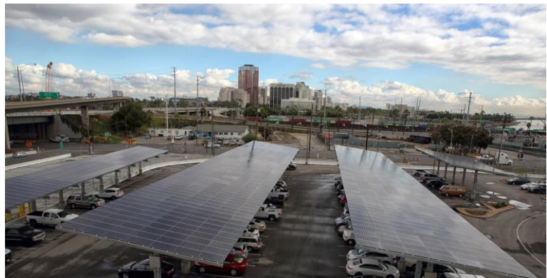
The 3,290 Mitsubishi Electric solar panels cover carports at Long Beach Container Terminal. Photo credit: Glen Marzano
